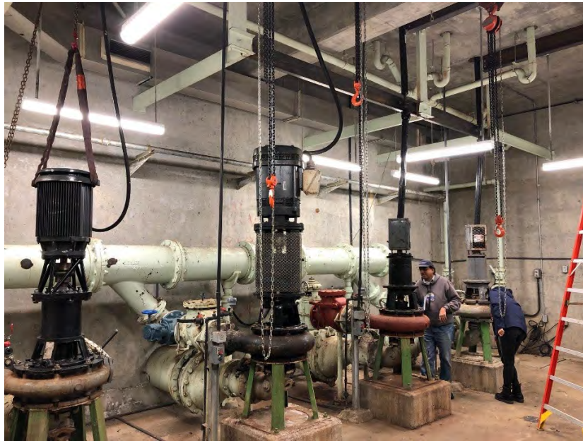
Pumps 1, 2, 3, and 4 (from left to right)
