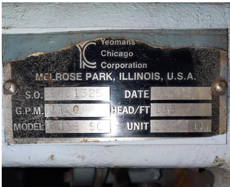
Figure 6. Nameplate of one of the existing shaft-driven pumps at PPS
