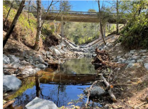
Post-construction photo of the Cloverdale Road bridge and stabilized Butano Creek channel bed.
