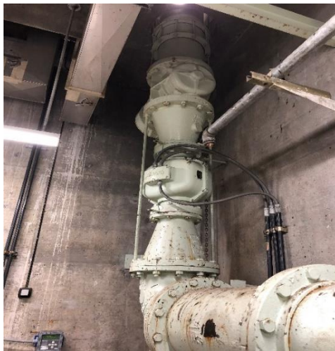
Figure B-4 Portola Pump Station Flow Meter
