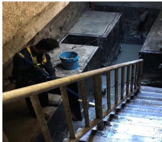
Figure B-5 Portola Pump Station Wetwell
