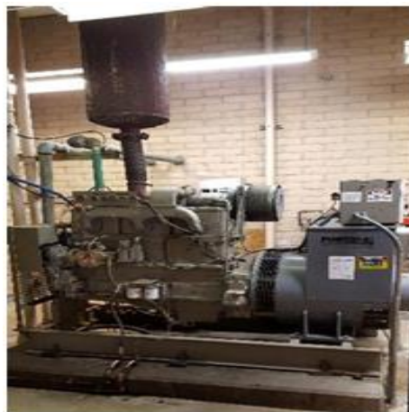
Figure B-3 Portola Pump Station-Generator
