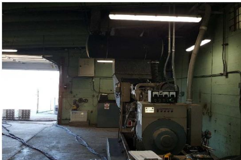
Figure B-1 Montara Pump Station Generator
